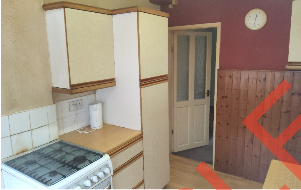
FIGURE 7 Chimney breast missing within the kitchen.
