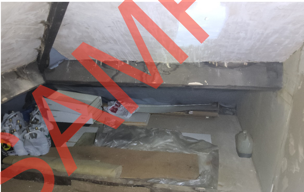
FIGURE 8 Poorly supported purlins with stains and cracking.
