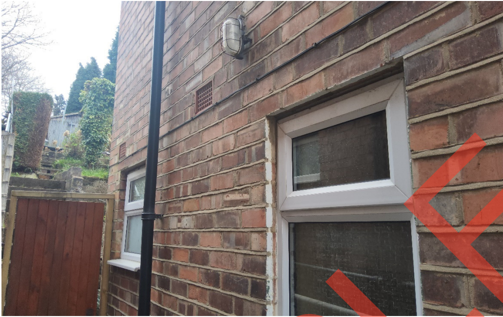
FIGURE 5 Lack of lintols above windows.
