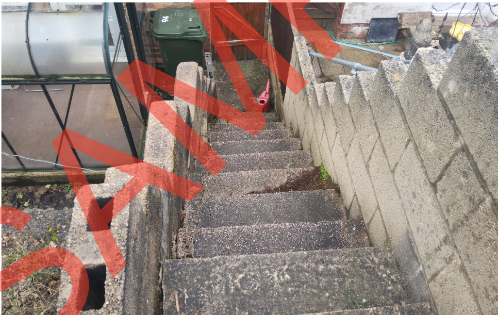
FIGURE 6 Distorted blockwork wall to the garden stairs.
