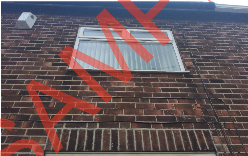
FIGURE 4 Cracking above the lounge window.
